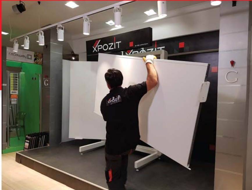
The lightweight magnetic panels are being installed onto the metallic structure in no time.
