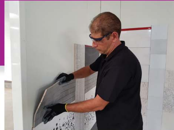
The last tiles are being installed - the system works very well with all tile formats. In the picture, the worker is installing mosaic tiles.
